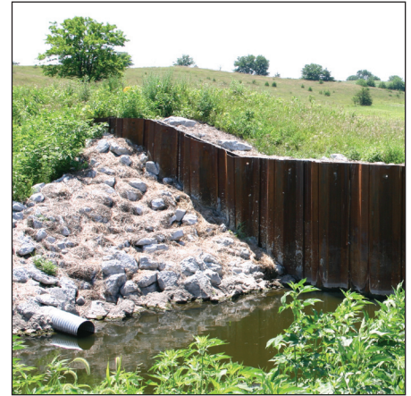
Water control structure constructed for treatment wetland project in Boone County, Iowa.
