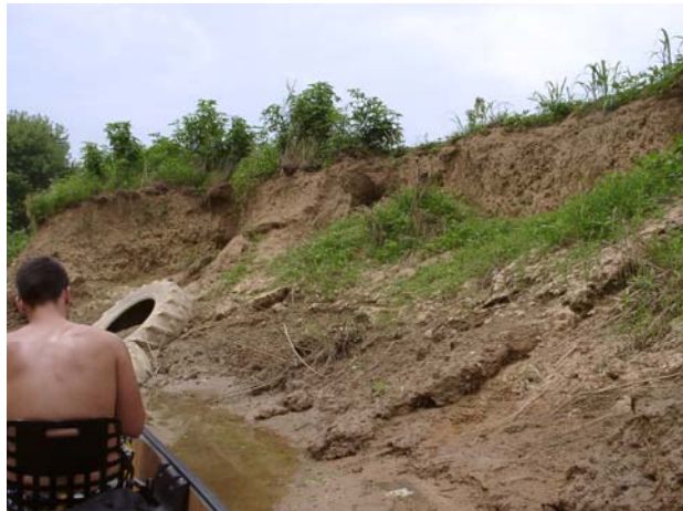
Green River bank with slump. Photo courtesy of J. Meiman
